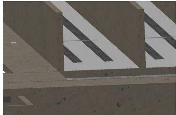
Photo 7 - Baseplate embedded in the bay floor
