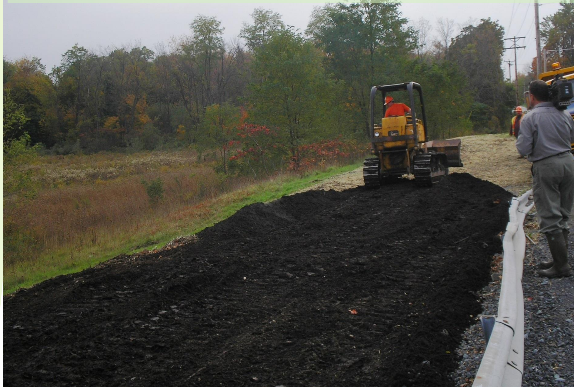
Roadkill compost spread Nov 2006 Highland NY DOT
